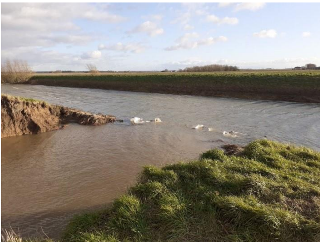
Photograph 1: Timberland Delph breach November 2019
