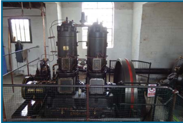
7: GAYTON ENGINE PUMPING STATION, Gayton le Marsh, off Gt Carlton to Theddlethorpe Rd., near Louth, LN12 1PE
