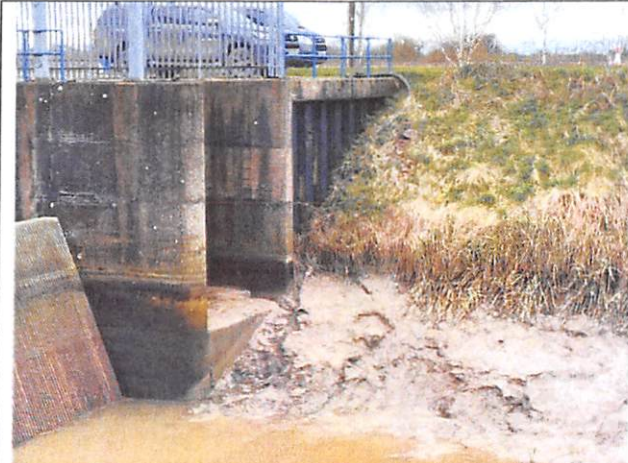
Photograph 7: RNS wing wall – pile section mostly buried
