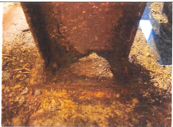
Photograph 5: Stanchion at lower slab level – hole
