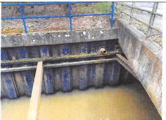
Photograph 6: Outfall - corrosion to steel bracing
