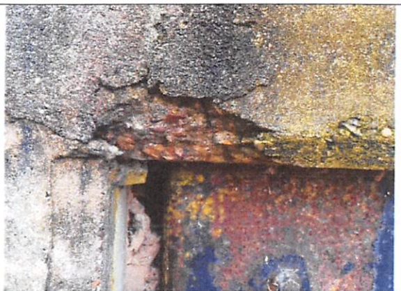
Photograph 4: LHS capping beam - localised spalling
