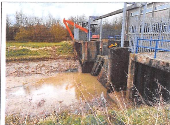
Photograph 1: Pumping Station Inlet
